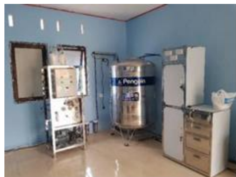
Gambar 13. Unit Reverse Osmosis
